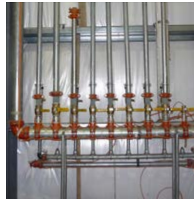
Fire protection systems
